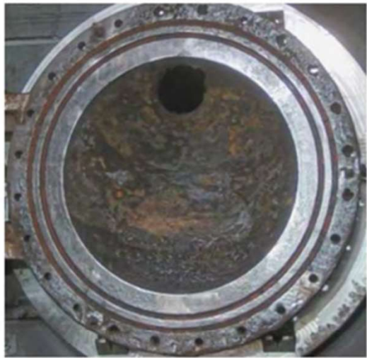
X-6 Penetration Before Cleaning
