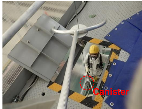
Capturing images of the canister being lowered to the first floor of the temporary house, from the second floor.
