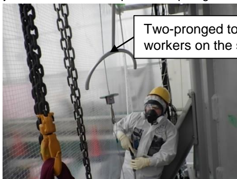
After storing the canister into the transport cask, separating the hoisting accessory
