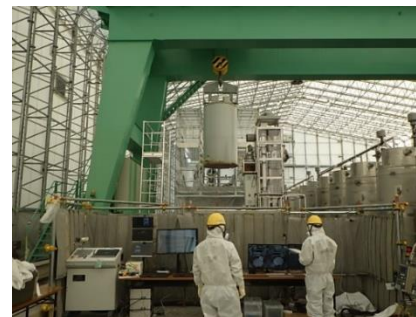
Figure 3 Verification of interference with the crane equipment
