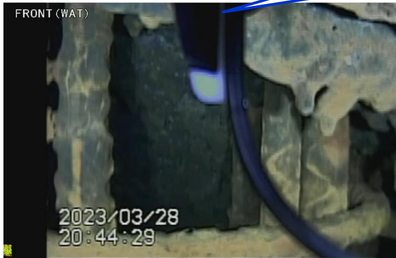
Photo 1: Concrete remains seen from the pedestal opening
