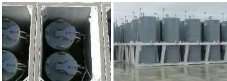
KURION adsorption towers SARRY adsorption towers No. of towers: Approx. 800 units No. of towers: Approx. 200 units
