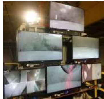
Monitoring of extension pipe-S/C surface with monitoring tool (No.7)
