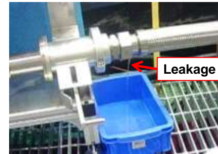
Example of leakage
