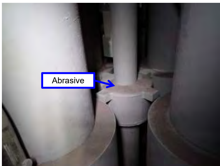
Deposit on the flange
