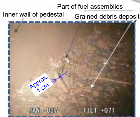
Results of investigation inside PCV of Unit 2 Photo of the pedestal bottom
